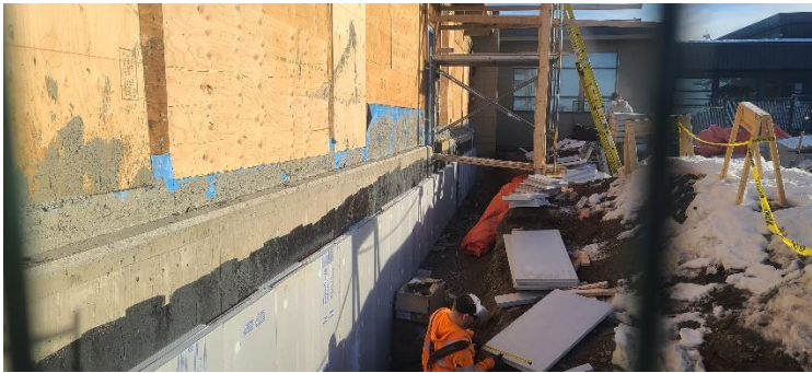
Subgrade insulation on the S side. The top 24" will be decorative Concrete Faced Insulation that will give a finished look to the visible foundation.
